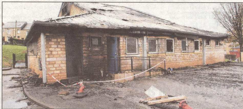
■ DESTROYED: The remains of the Thornton Lodge Community Centre after the fire this weekend
